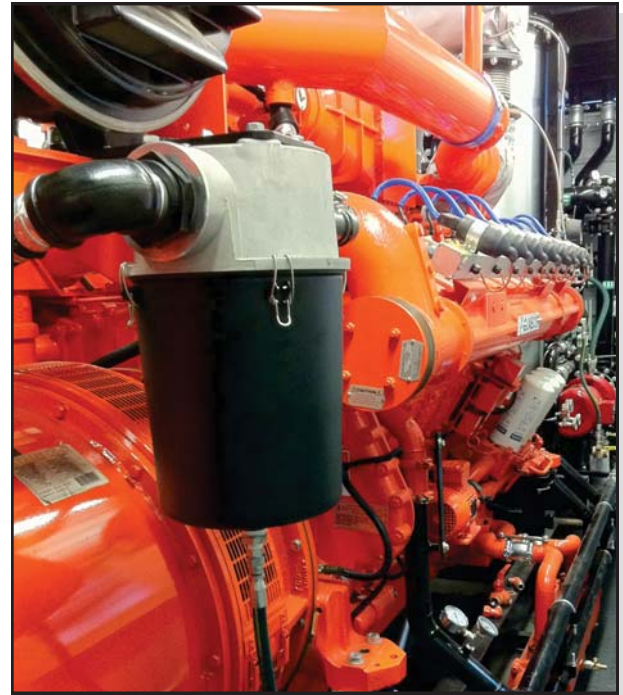
Closed Crankcase Ventilation System Guascor Engine Installation
